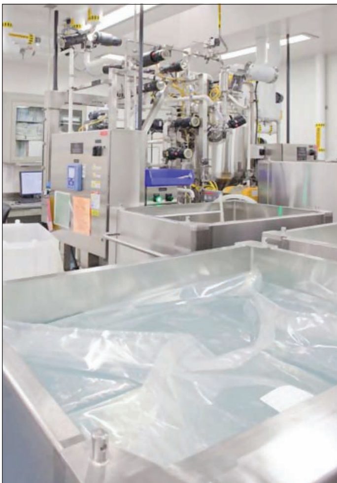
Mid volume buffer tote for UF operation.
