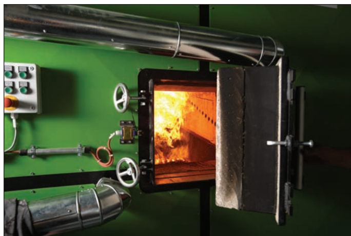
Wood pellet steam boiler.
